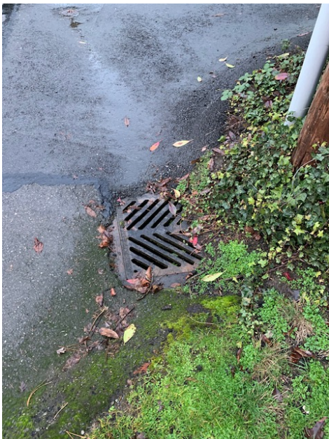
Catch Basin – At Point B
